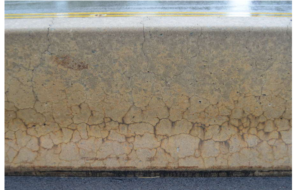
Figure 2: Cracking due to ASR
